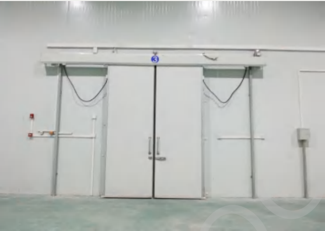
Electric sliding door
